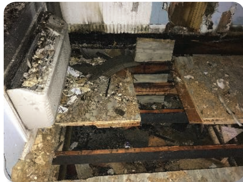
Electrical heater in basement of unit 705 where the fire started.
